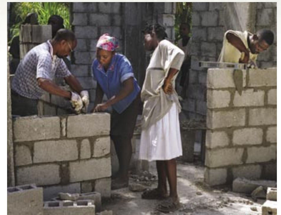
Pastors Oniel Saint Louis and Asquin Astrel are aided by local women as they construct the interior walls of the ministry home in Maillette.
